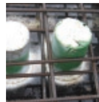
Cracked and broken Sleeves
