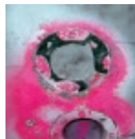
Concrete filled sleeves
